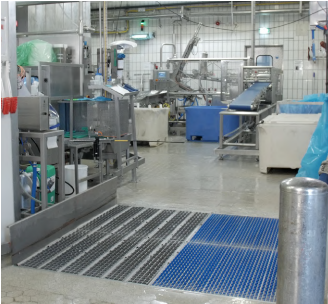
Installation in a dairy plant
